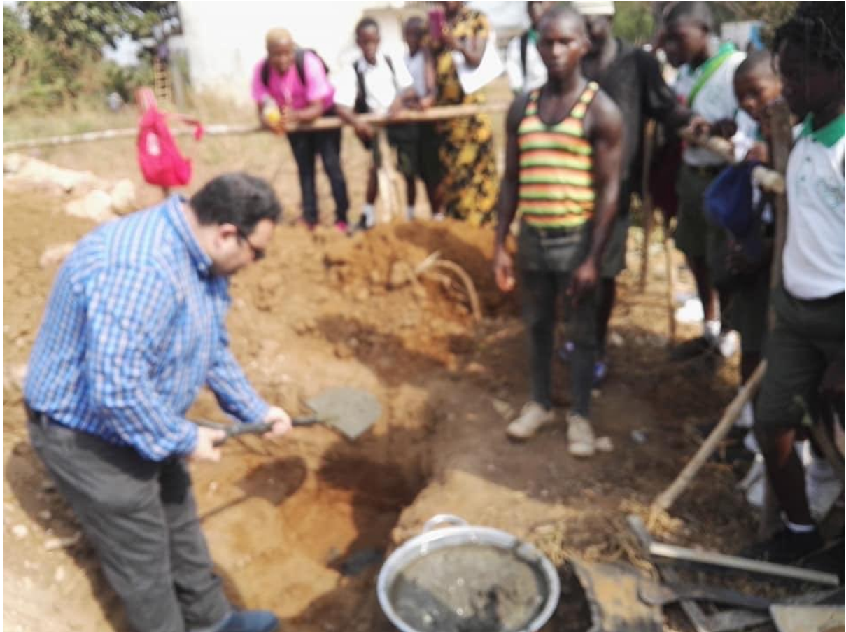
VICE CHAIRMAN BOARD OF DIRECTORS SIERRA LEONE CRICKET ASSOCIATION MARTIN MICHAEL TURNING THE SOD FOR THE CONSTRUCTION OF THE PRINCE OF WALES SCHOOL CRICKET GROUND 300 SEATER PAVILION.
